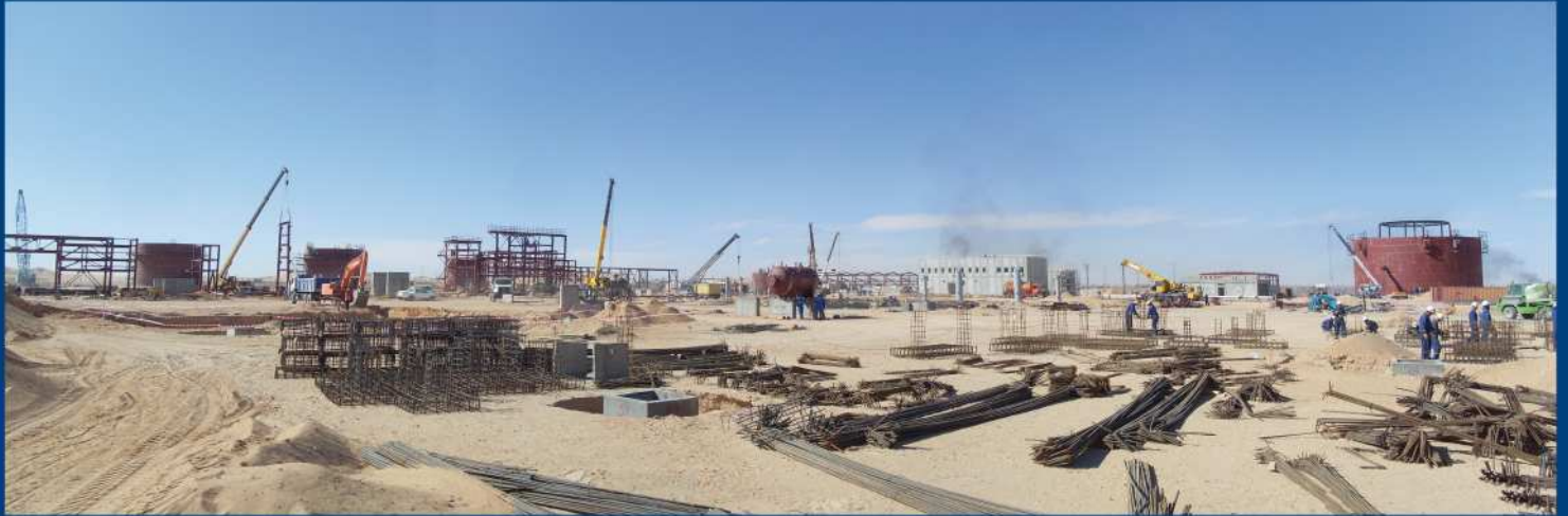
Oil and gas processing plant - RHOURE-NOUSS
